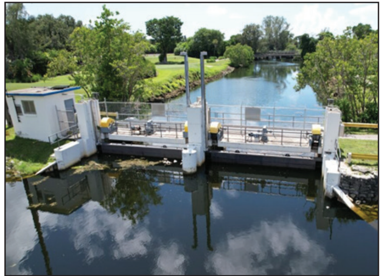
S-28 Structure Gate.
