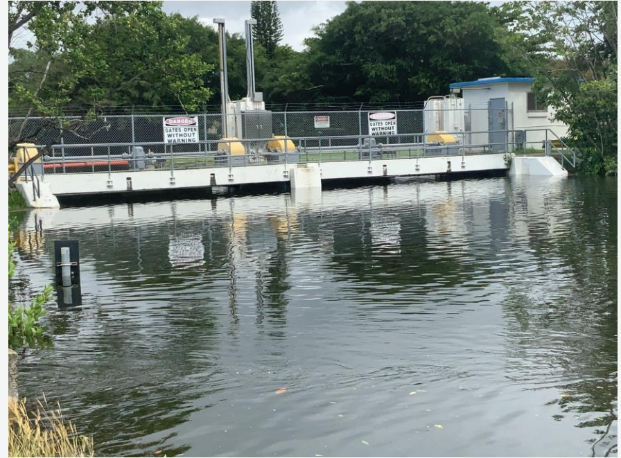
Photo: High tailwater observed at S-28 Spillway Structure on October 08, 2025 (Looking Upstream from Downstream)
