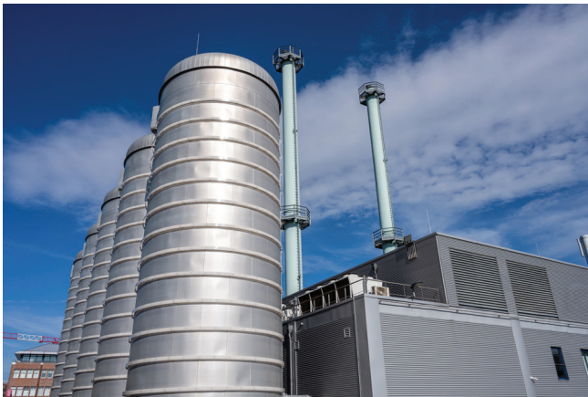
Combined Heat and Power Generator
