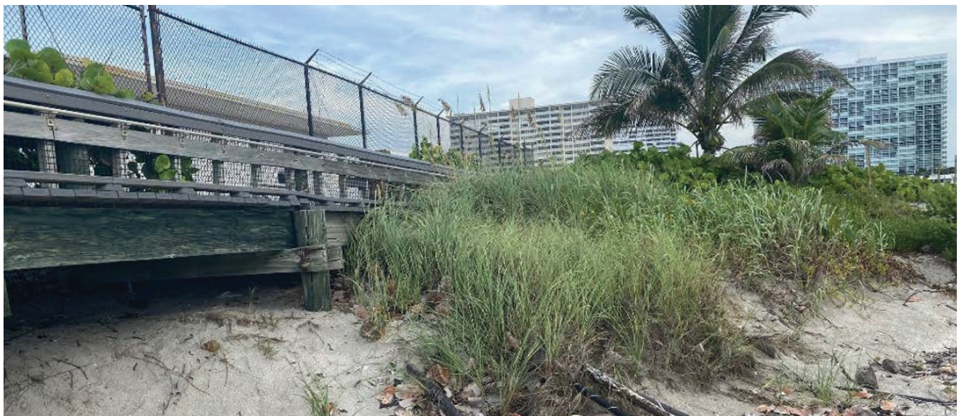
Shoreline Erosion and Damaged Jetty
