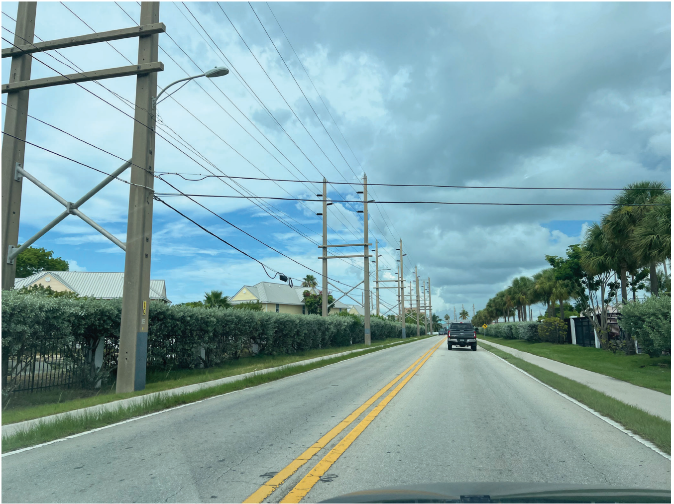
Power Infrastructure at NASKW
