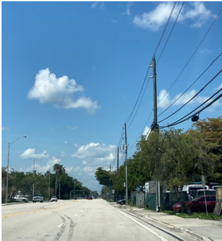
Wood Utility Poles
