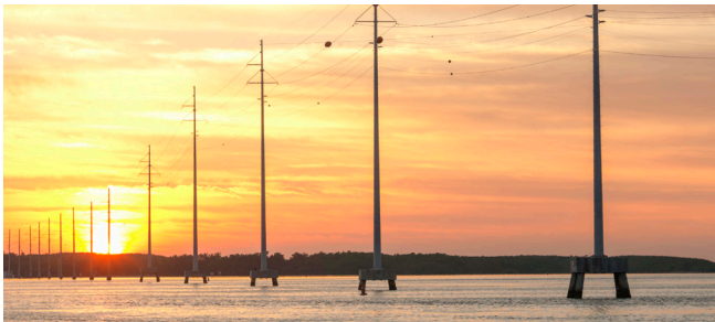
Electrical Power Lines Servicing Key West
