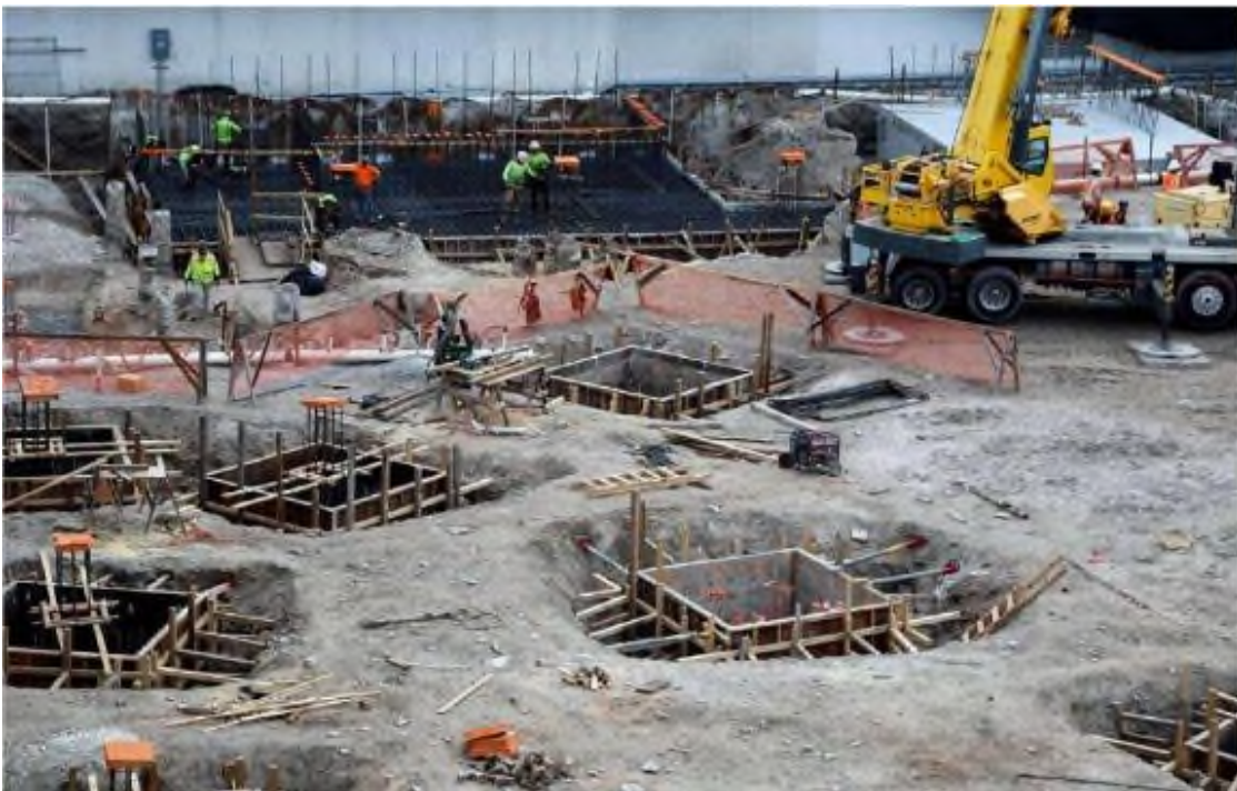
Construction on a $500 million multi-year project is underway at the Bal Harbour Shops in Bal Harbour, Florida, on Wednesday, January 10, 2024. Al Diaz adiaz@miamiherald.com
