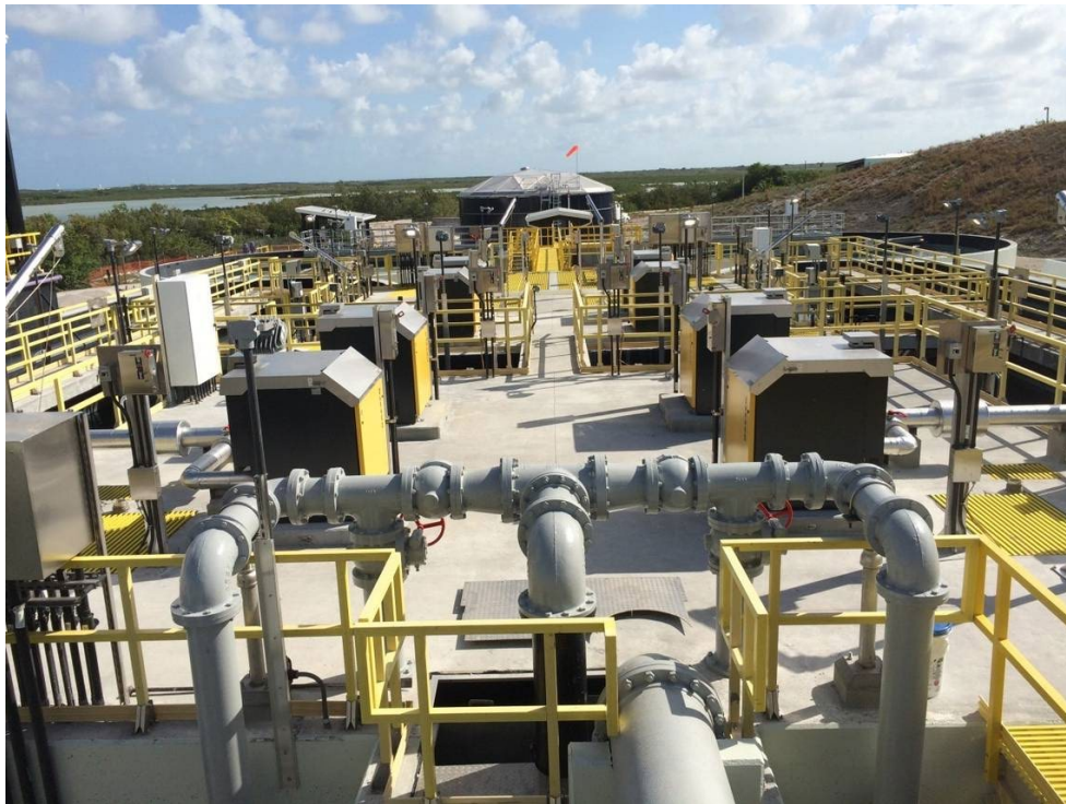
This is the Cudjoe Key sewer treatment plant.
