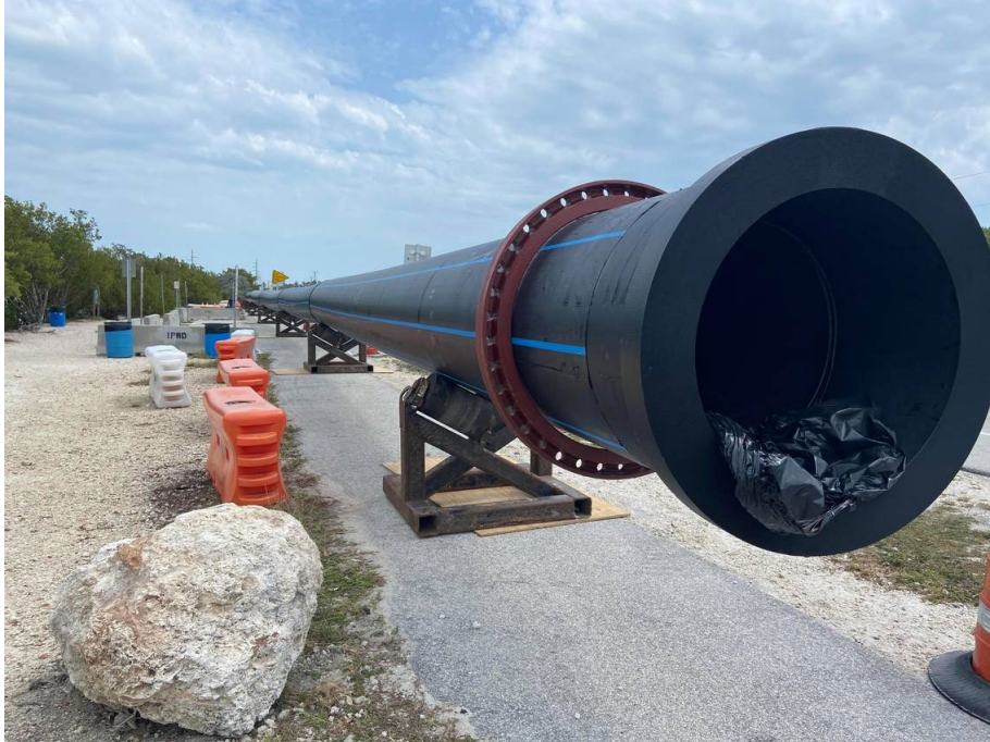
Water pipes are propped up on the side of U.S. 1 at mile marker 79 in the Florida Keys Tuesday, March 14, 2023. The pipes are part of a $42-million project to replace aging infrastructure in the Upper Keys. David Goodhue/dgoodhue@miamiherald.com
