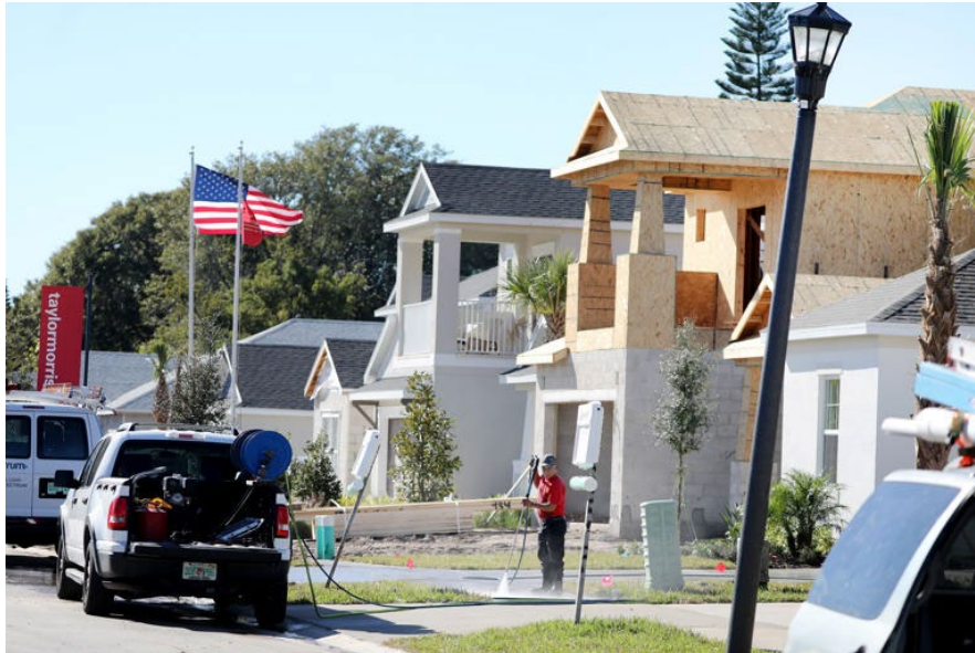
A worker pressure-washes a driveway at a new home in the Silver Ridge subdivision under construction in Palm Harbor on Dec. 28. Florida led the nation in population growth in 2022, and economists with the Florida Chamber of Commerce believe millions more will arrive in the next few years, buoying the state's economy if the U.S. enters a recession. / © Douglas R. Clifford/Tampa Bay Times/TNS
