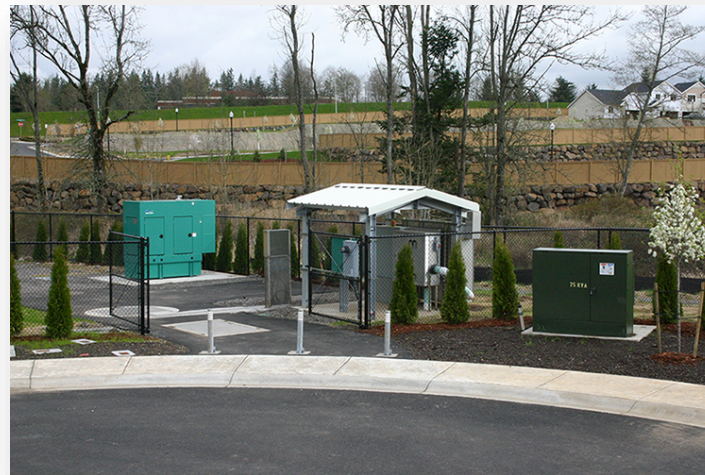
Underground Pump Station Injection Well (No Pump Station building)
